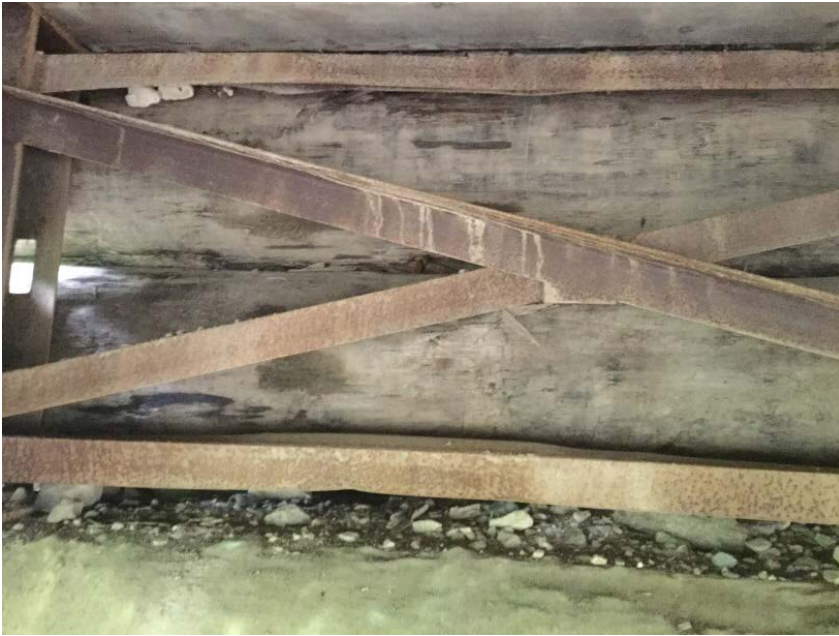
Slight damage to right bank diaphragm
