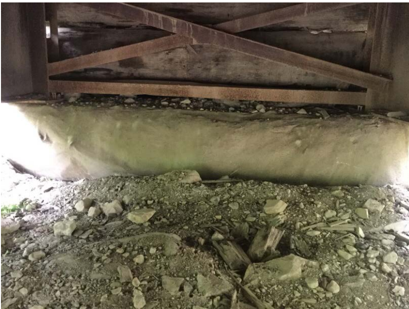
The girders do not sit square on either log sill
